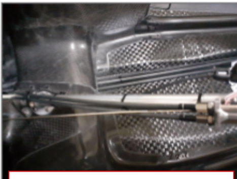
B12.1 Cables must be well secured
