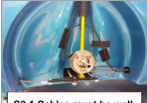
C3.1 Cables must be well secured
